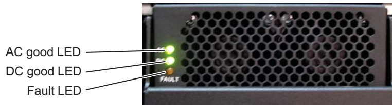
Figure 3-6. Power Supply LEDs
